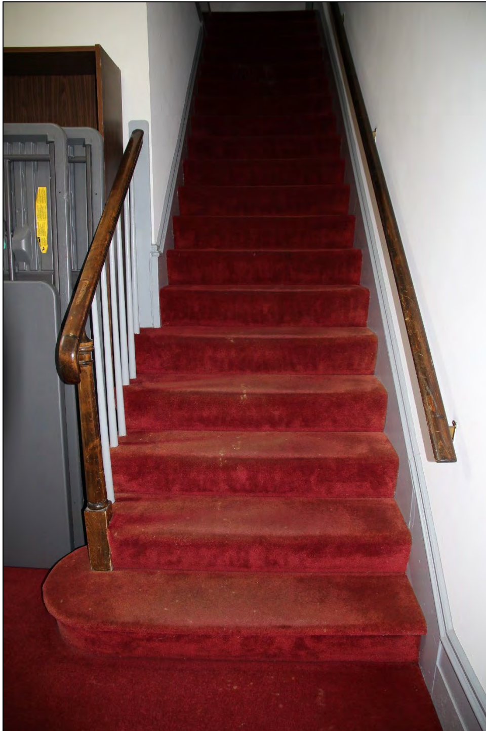
PHOTO 27: View of Staircase to Second-Floor Conference Rooms and Bathrooms (N. Holst, August 29, 2022)
